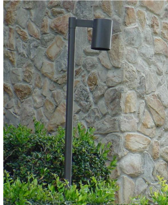
Arm-mounted downlight on pole along walkway.
